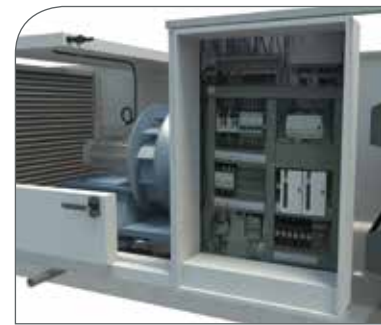
Segregated cable channel and factory-installed control panel
